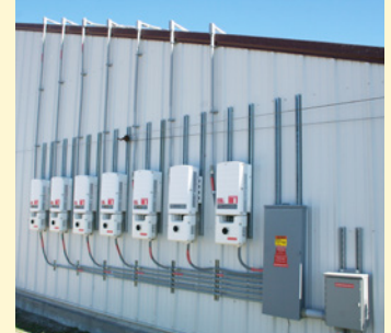
▲ A set of string inverters
