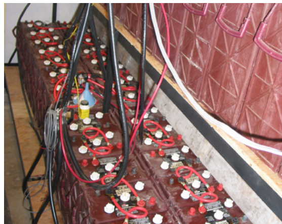
▲ A battery bank
